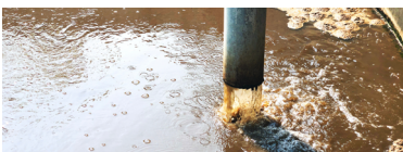
Leak & Discharge Monitoring
