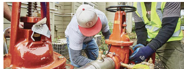
Backflow Prevention and Cross Connection Control
